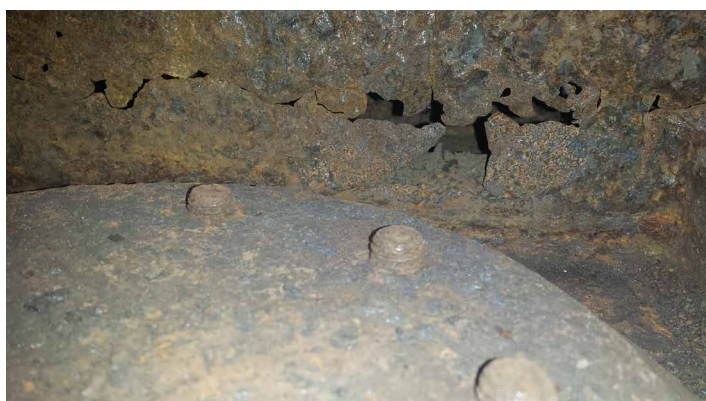
On closer inspection, severe corrosion was identified around the skid plate support structure
